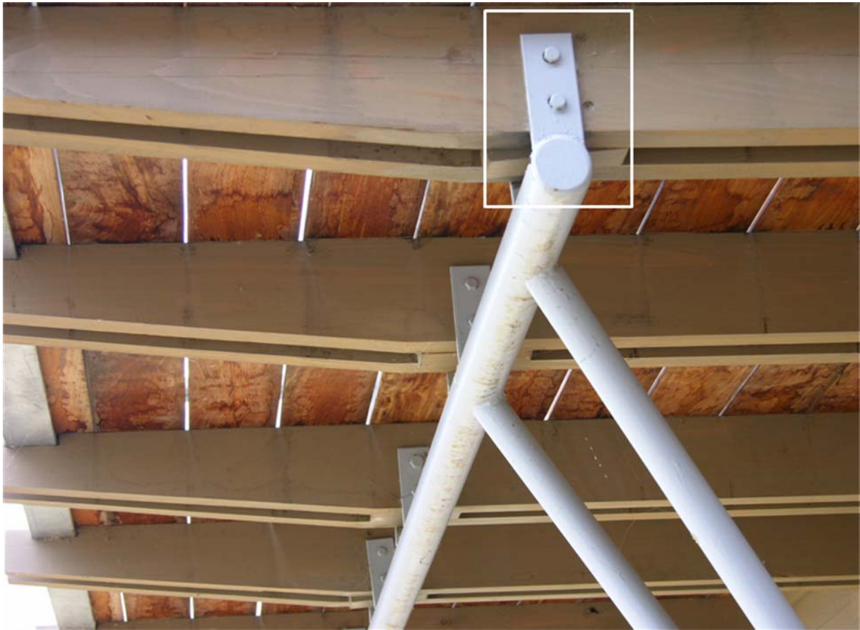
The conduit clamps have been replaced by welded clamps, which were originally called for in the plans.
